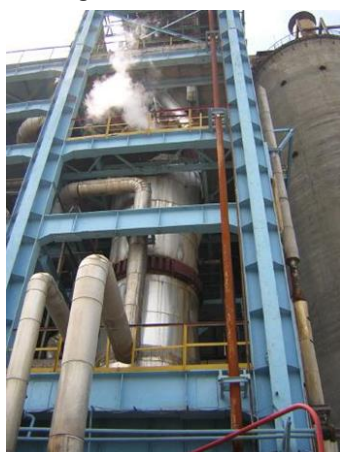
Urea stripper in Romania
