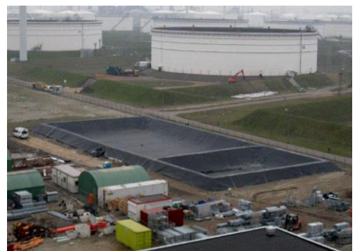
An effluent pit after the earthworks (top) and the final result (bottom)
