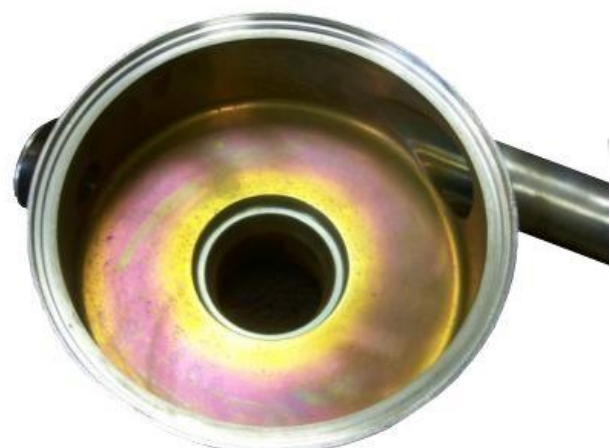
Pump casing with rouging before treatment
